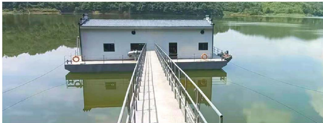
浮船式取水泵站 Floating Water Intake Station
