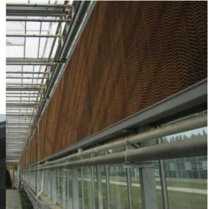
Evaporated Pad Wall
