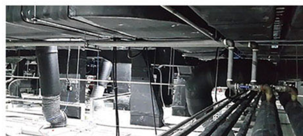
Ventilation duct system1/2
