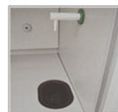
Water Tap & Water Sink
