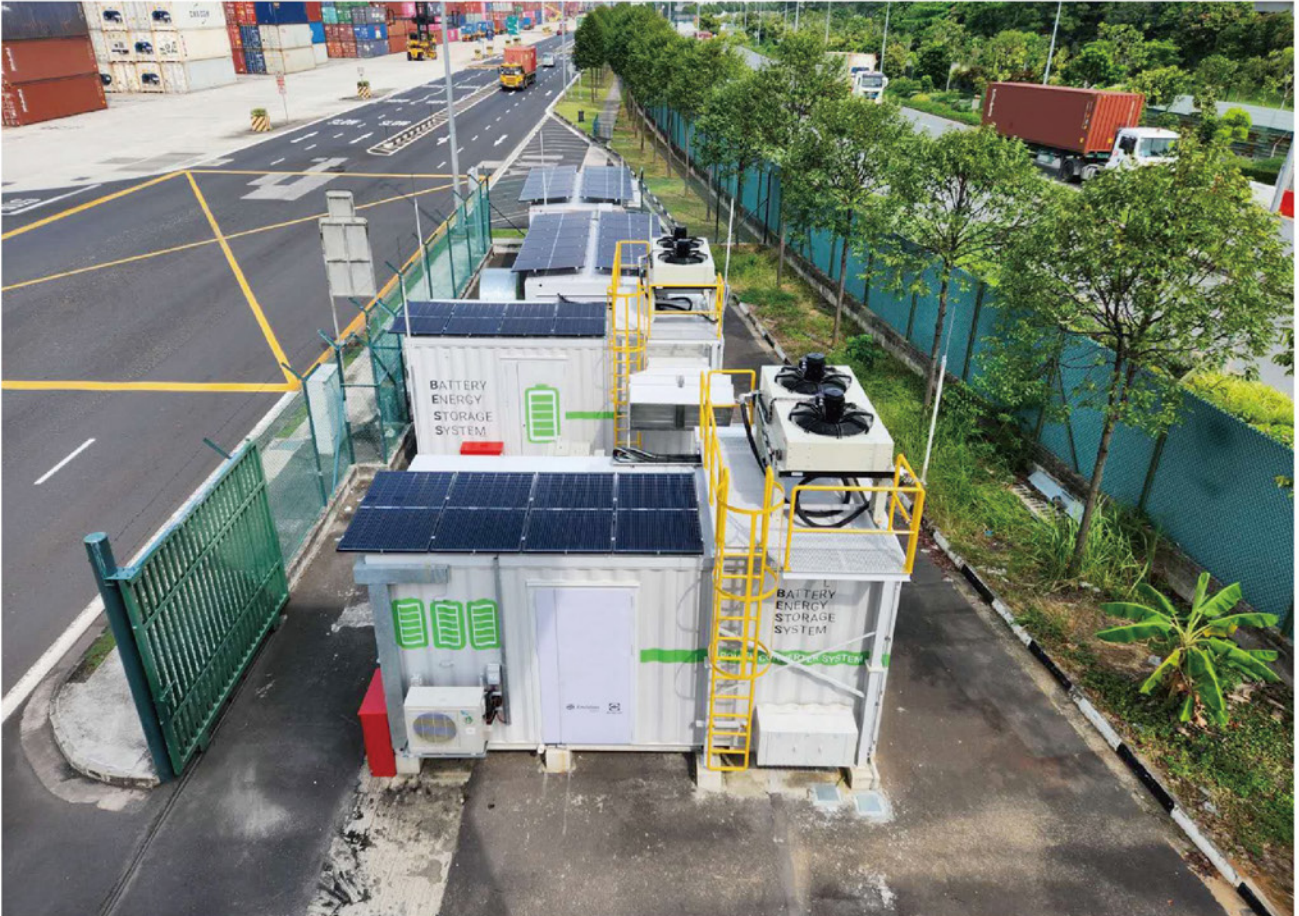
▲ 2MW bi-directional DC/DC converter Singapore
