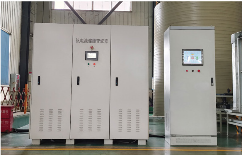
◀ 1MWH Vanadium battery energy storage system Hunan
