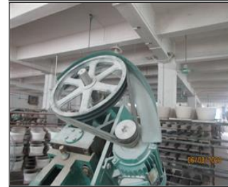
External photo(s) of the production unit(s) NC 7.17 No pulley guard.JPG
