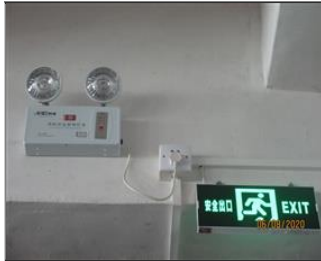
External photo(s) of the production unit(s) Emergency light and exit sign.JPG
