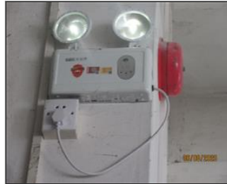
External photo(s) of the production unit(s) Emergency light testing.JPG
