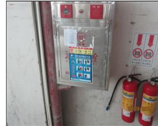
External photo(s) of the production unit(s) Fire hydrant and fire extinguishers.JPG
