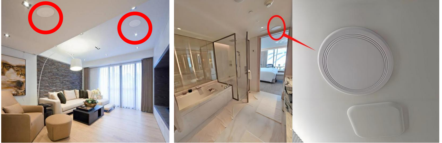
KBT Antennas Deployed at Residential Buildings
